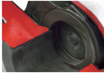
Inside of Gate valve
