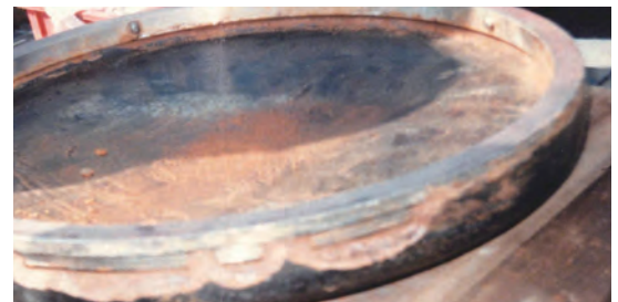
Disc of a swing check valve that has been corroded by seawater
