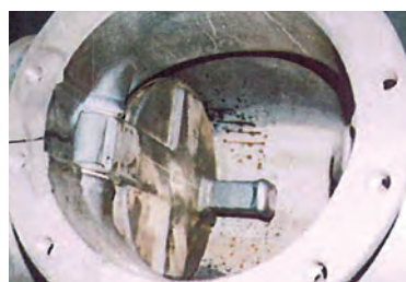
Inside of Swing check valve
